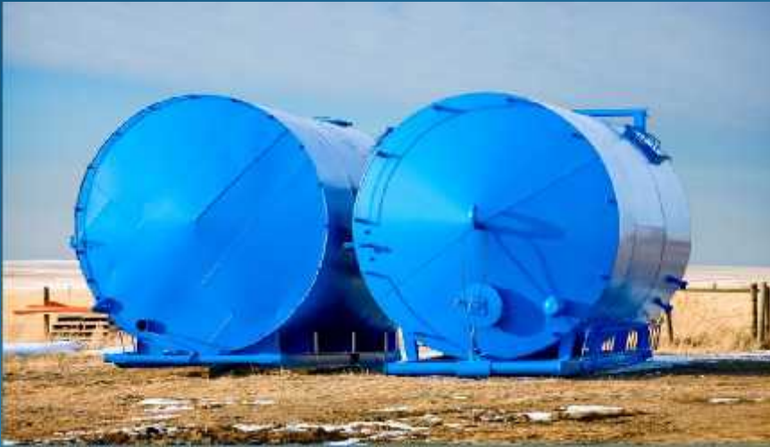
Oilfield Storage Tanks
